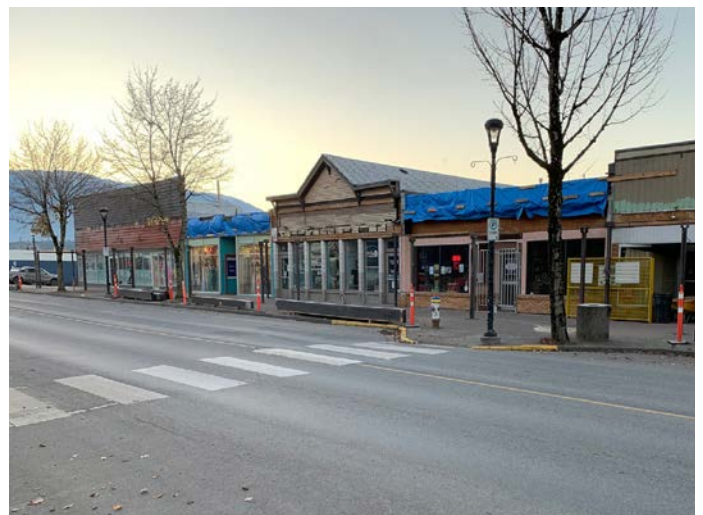
Right: The removal of the 4600 block of Lakelse Avenue sidewalk canopy began in September 2023. The work is ongoing in 2024. Staff have also been working with TDIA on a conceptual design for the redevelopment of the 4600 block of Lakelse Avenue.
